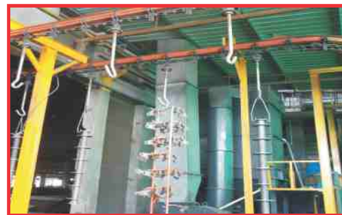
Conveyorized Paint Shop
